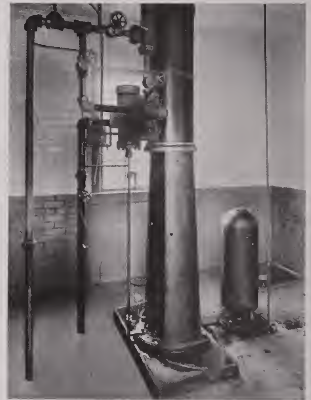
COOK DEEP WELL PUMP
